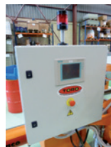
Electrical Control Panel
